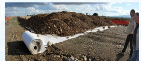
Installation of a draining geocomposite at the base of the railway embankment. In this case the GCD is installed across the embankment
