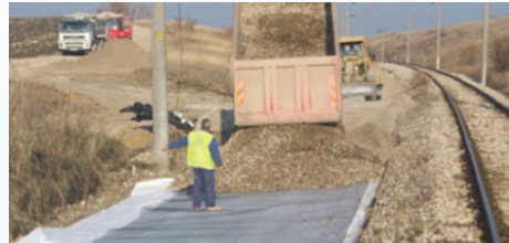
Geotextile – geogrid geocomposite laid directly on the soft subgrade for providing separation, filtration, and stabilization
