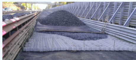
Combined use of geocells, geogrids, and nonwoven geotextiles for stabilizing railway tracks
