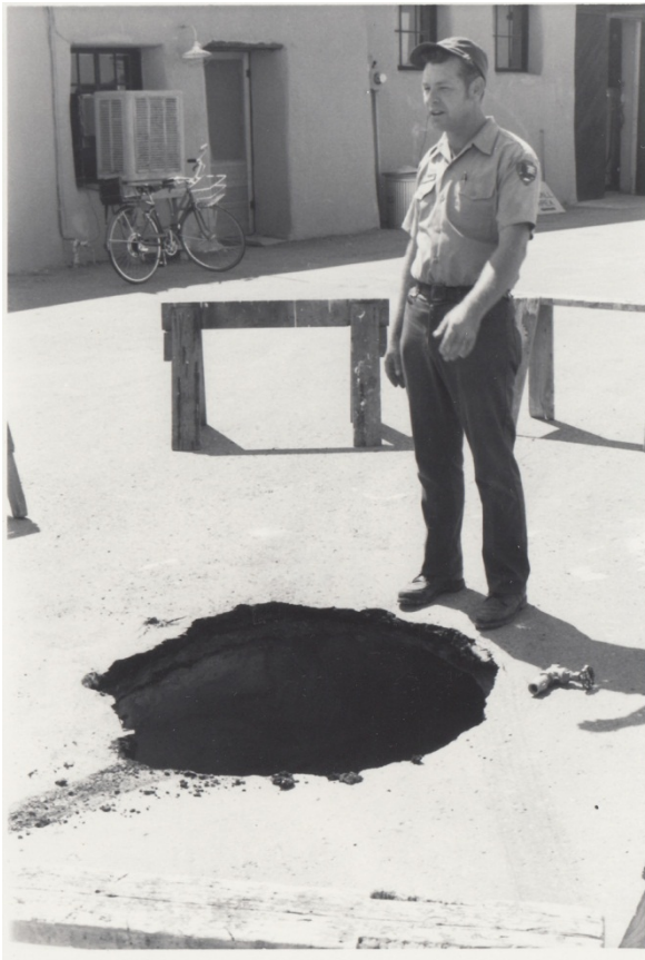
Figure 14. Sinkhole. Because gypsum readily dissolves in freshwater, leaky water lines can cause dissolution and collapse. Collapse occurred, creating a sinkhole, in the maintenance area parking lot at White Sands National Monument in 1975. National Park Service photograph.
