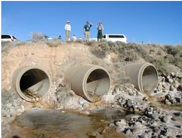
Figure 9. Culverts at White Sands Missile Range. Changes in natural drainage patterns, for example by raised roadways and culverts at White Sands Missile Range, have changed surface water flow and exacerbated erosional processes, threatening archeological resources in adjacent White Sands National Monument. Photograph by Katie KellerLynn (Colorado State University), taken by permission during the 2003 geoindicators meeting.
