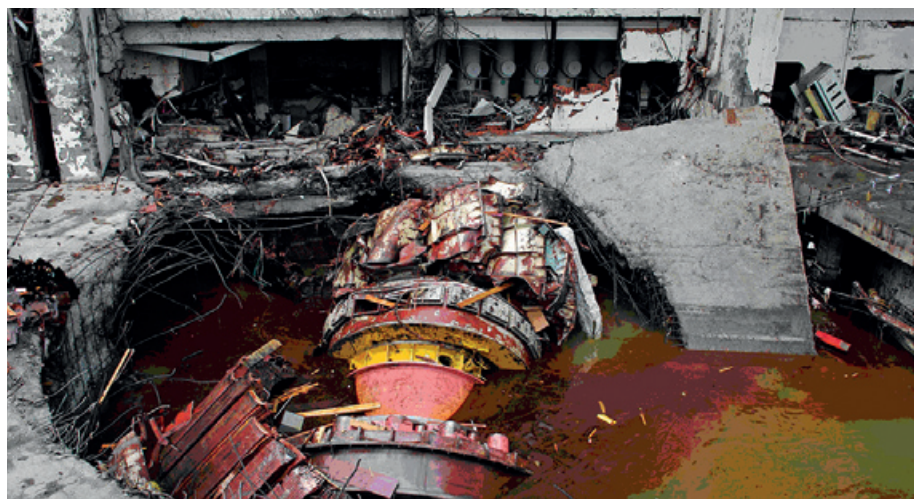
Figure 5. Unit 2 several hours after failure.
