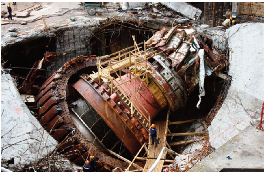
Figure 2. Part of the damage to the powerhouse after the 17 August 2009 accident. Unit 2 as seen on 3 September 2009 after dewatering.
