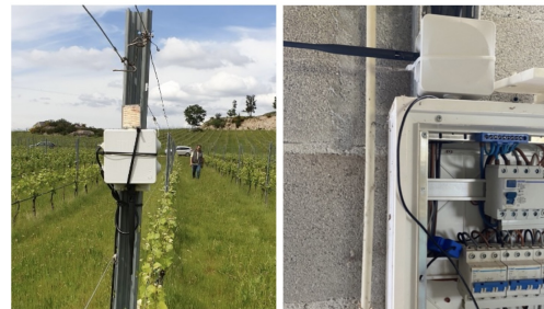
Fig. 6. IoT nodes installed in the case study.
