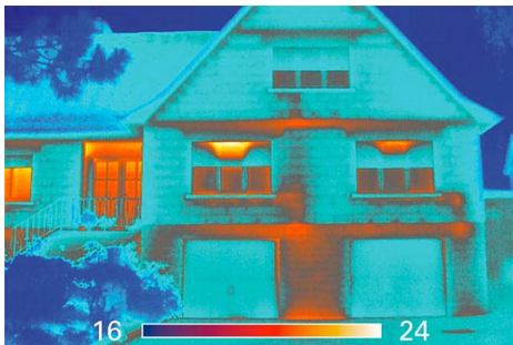
Fig. 9 Thermal image of a building, showing a higher amount of heat loss around windows and doors [149].
