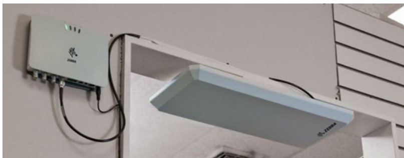
Figure 2-6 Fixed doorway RFID reader
