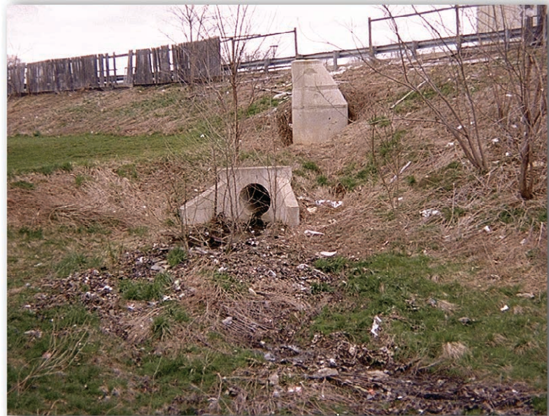
Storm water in a city is usually collected in storm sewers and transported to a stream in large pipes. This photo shows water exiting a pipe into a stream.
