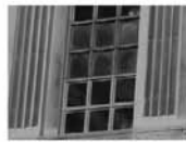
FIGURE 11 Exterior before (top two rows) and after (bottom two rows) view showing original windows and blast resistant replicas illustrates minor muntin-voiding needed to secure the thicker laminated glass of the new blast window. (Mariah McGaughey/GSA)
