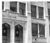
FIGURE 10 Exterior view of blast windows fabricated with custom muntin placing upper and lower panes in separate planes to simulate the appearance of double hung windows. (Mariah McGaughey/GSA)
