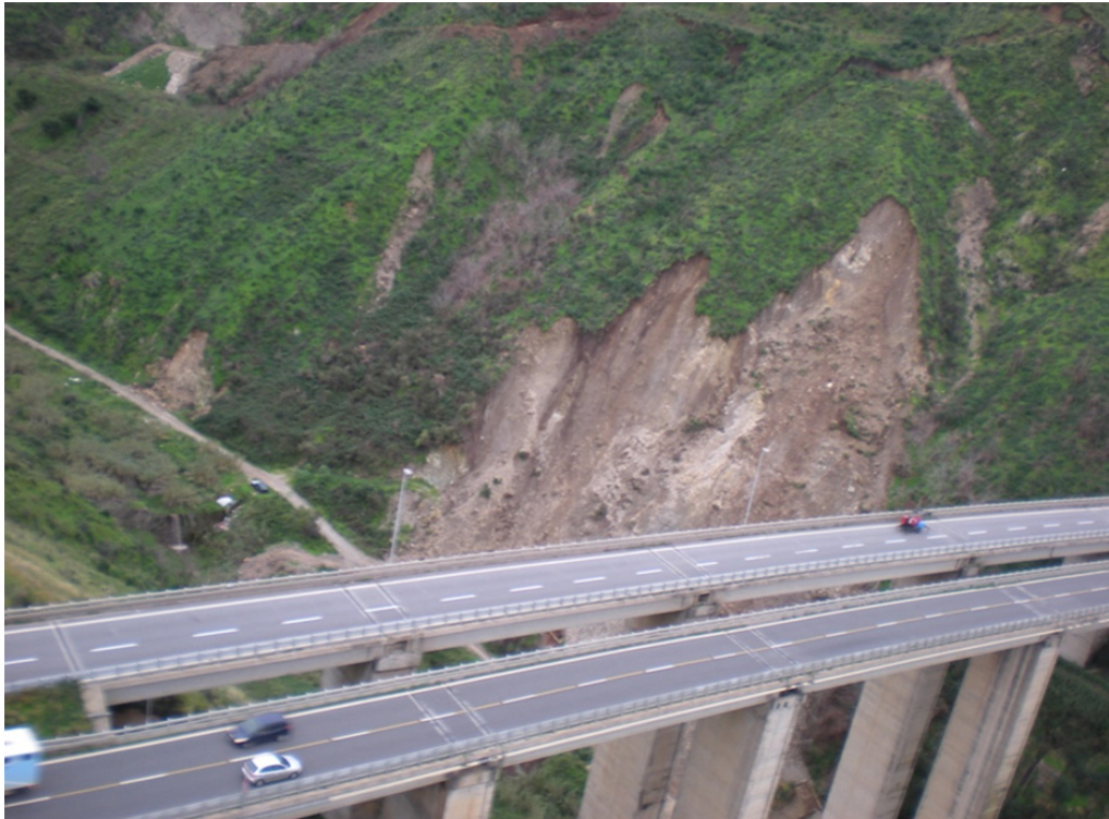
Fig. 2. Picture of Santa Trada landslide nearby the viaduct of the A3 motorway.
