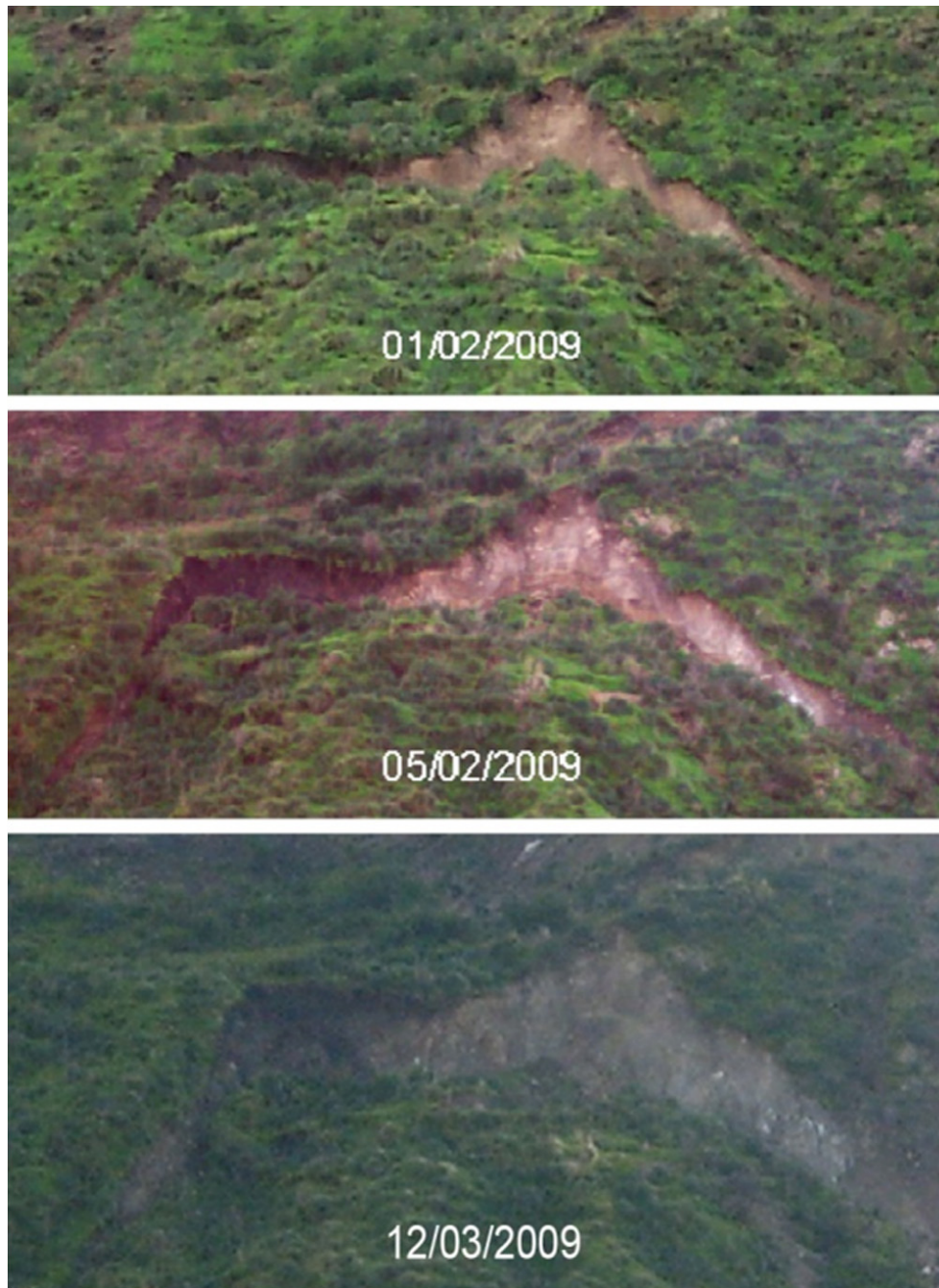
Fig. 3. Pictures of a fracture placed above the landslide. The widening of the fracture with time is clearly visible.
