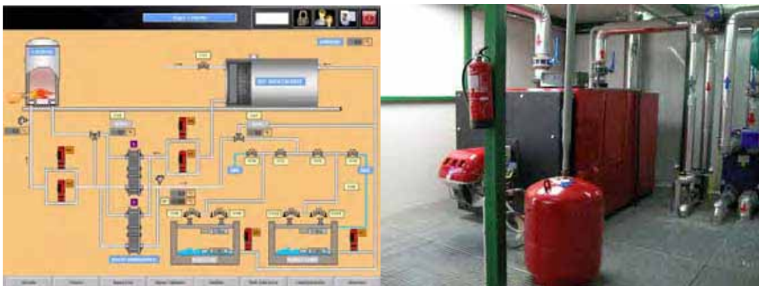
Hot water control system (left) and general view of boiler (right)
