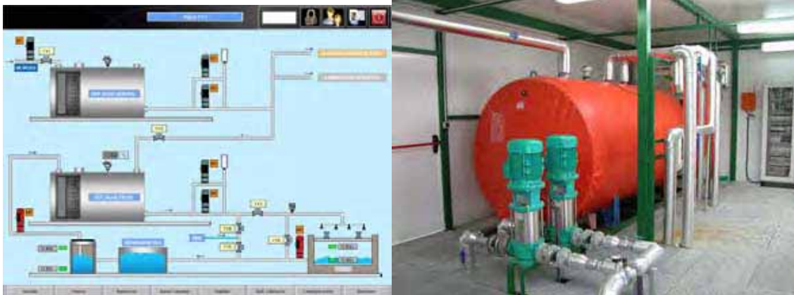
Control system (left) and general view of water installation (right)
