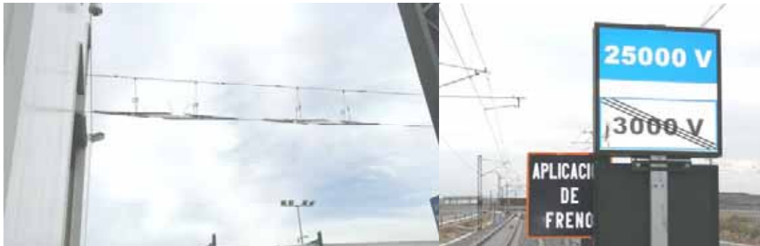
On the left, overhead isolating switches at the entrance to the changer. On the right, the signal shows the change in electrification voltage
