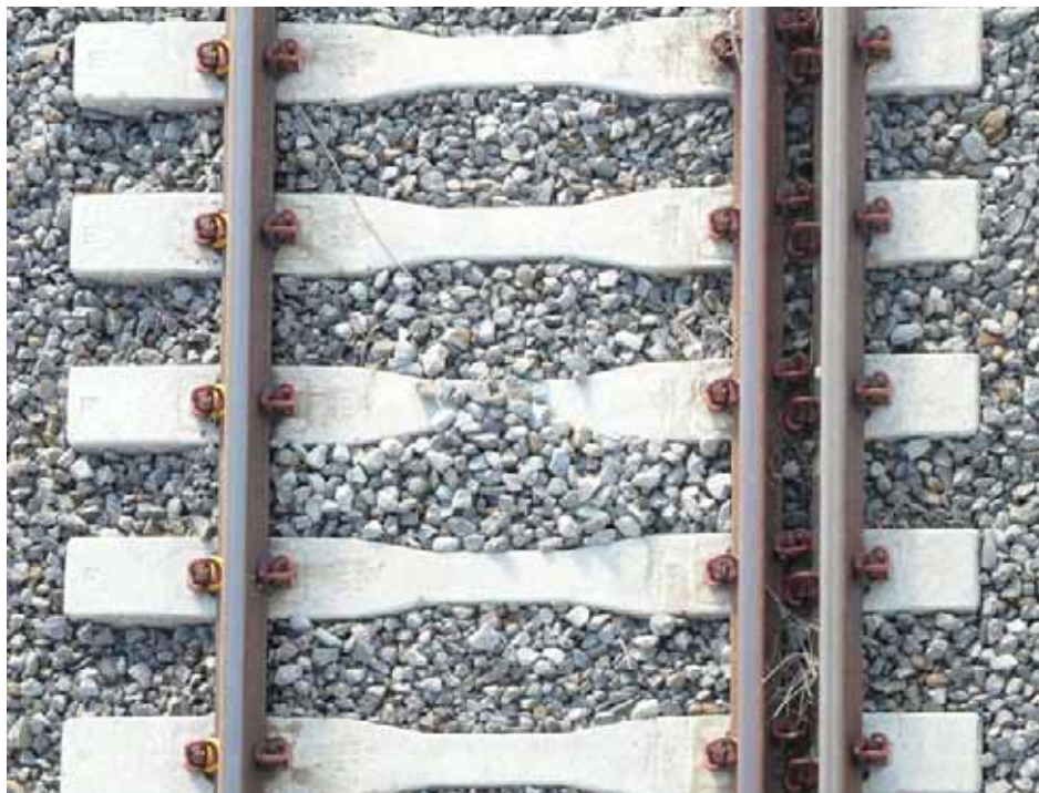
On the three-rail track we can see the difference between the standard gauge (1,435mm) and the Iberian gauge (1,668mm). The photo was taken at Pozal de Gallinas, on the Olmedo-Medina del Campo test section
