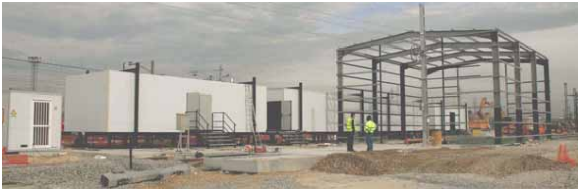
Portable modules containing the auxiliary systems are built next to the third generation changers
