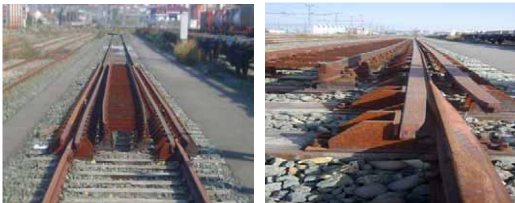
Changer for Rafil and SUV-2000 technologies installed at Irún for tests
